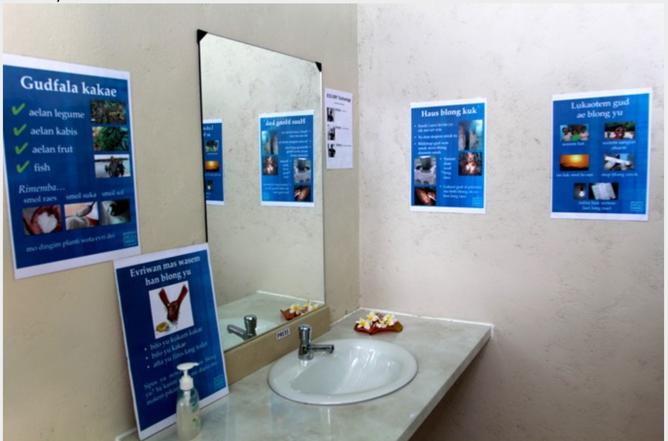
Two female toilets, two for men, and a disabled access were built by villagers. (Photo: Melinda Trochu)
